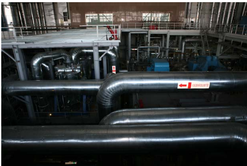
Figure 3 First heat exchange station for the heating system updating project located in Huaneng (Yingkou) Power Plant.
