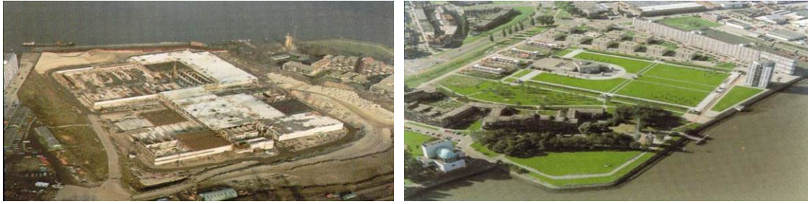
Figure 3: Dokhaven Waste Water Treatment Plant during construction (left) and after completion (right). Courtesy: City of Rotterdam
