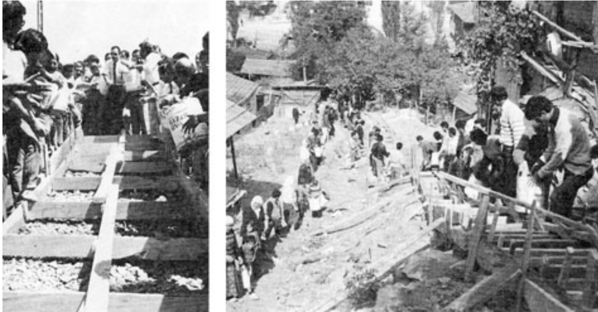
The Zafertepe inhabitants and members of the Cevre-Koop during the construction of one set of steps in their settlement (from Goksu, A. Faruk, 1996).
