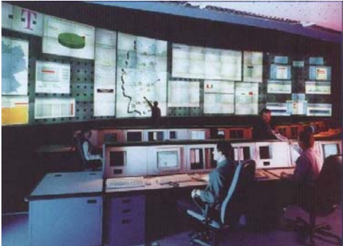
Telecommunication Net Management Center in Bamberg
